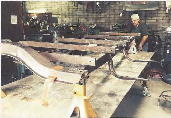
Local Model A Club members recommended that the frame should be checked for straightness and against factory tolerances, which is underway here. Any twisting would have to be corrected before work could continue, but the frame was found to be true.
